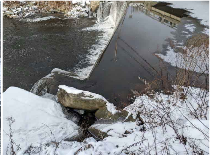
November 2021 – Flow through left abutment
